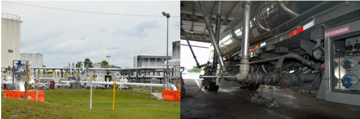
Figure 2: Fuel distribution terminal and tanker truck Image Source: AAA
